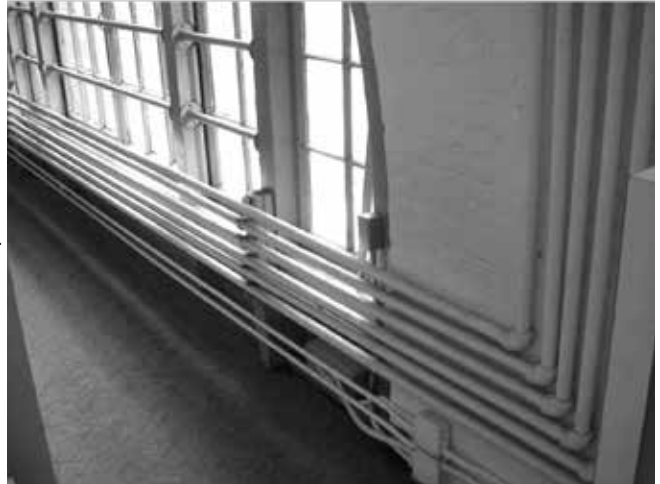
Figure 23: Hydronic System Piping
